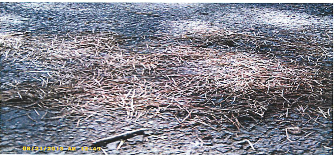
MORE PICTURES OF NEEDLES DROPPING AND OTHER SHEDDING FROM THE CEDAR TREE, CAUSING SLIPPERY CONDITIONS BELOW ON TARMAC
