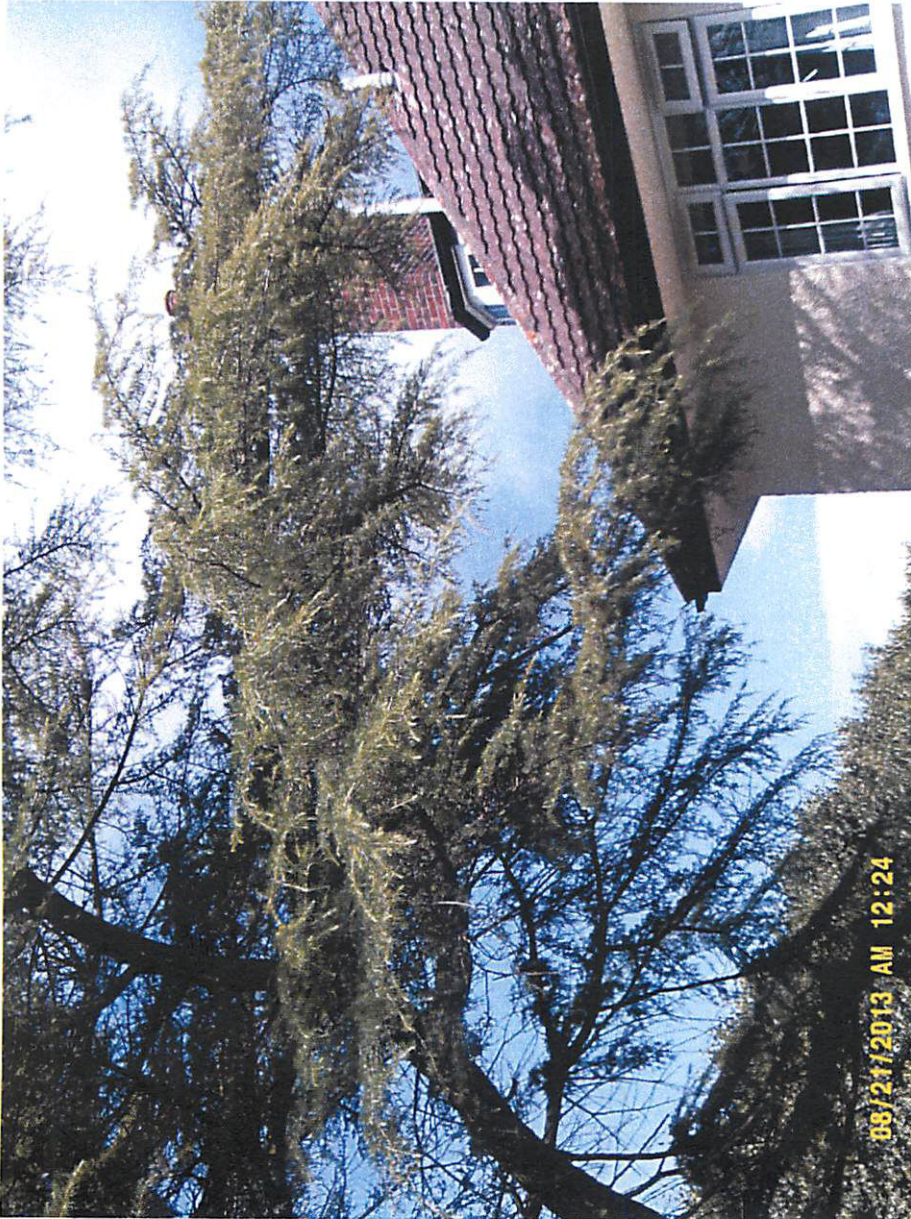
THIS LARGE BRANCH OF THE TREE IS IN CLOSE PROXIMITY TO THE BUILDING
